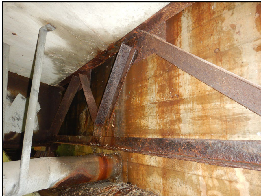
Photo 18 – Looking southeast at the end cross-frame between beams D and B at the Rear Abutment. Note: up to 1/4-inch section loss to the bottom strut angle.
