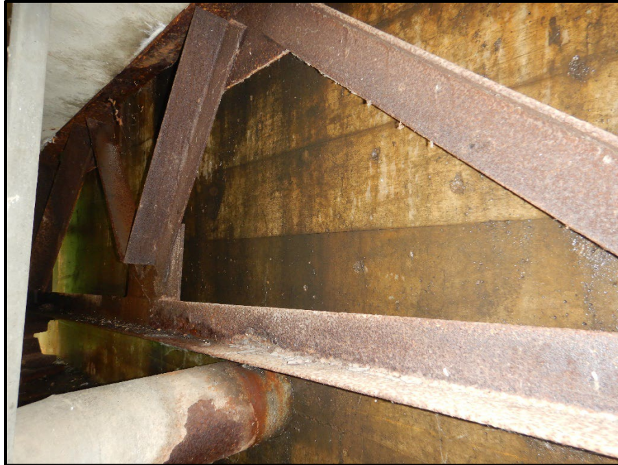
Photo 27 – Looking southwest at the water staining and cracking in the Rear Abutment backwall.
