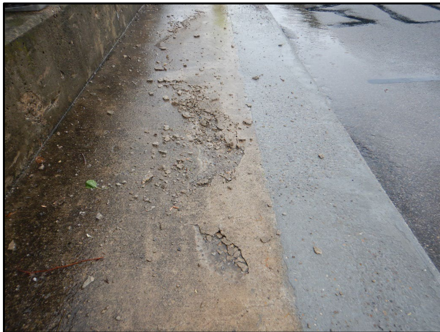
Photo 8 – Looking west at the south sidewalk in span 3. Note: 7-foot-long section of the sidewalk is scaling.
