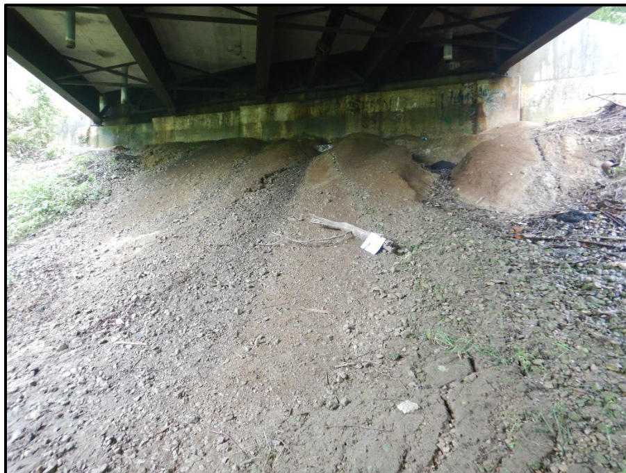
Photo 28 – Looking east at multiple erosion ditches formed by scupper drainage in embankment in front of the Forward Abutment. Similar conditions are present at the Rear Abutment embankment.
