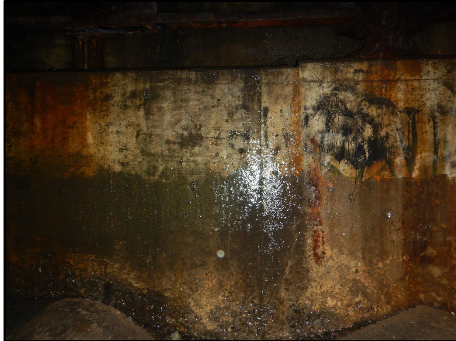
Photo 29 – Looking east at active water leakage down the Forward Abutment backwall.
