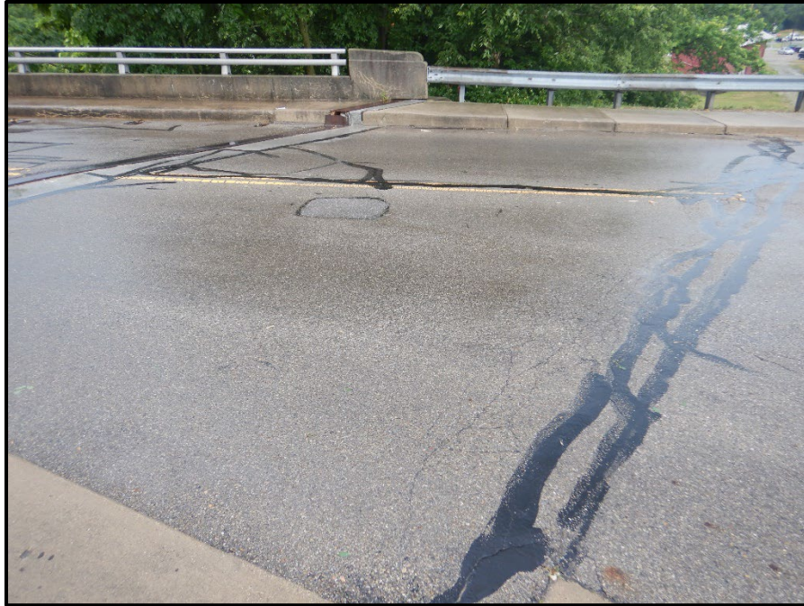
Photo 35 – Looking south at the west approach roadway. Note: multiple sealed transverse and longitudinal cracks in the approach roadway.
