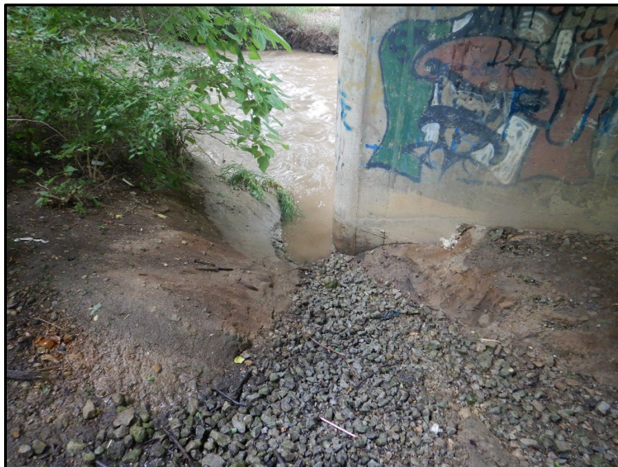
Photo 34 – Looking west at the scour hole at the end of an erosion ditch at the south end of the Forward Pier.
