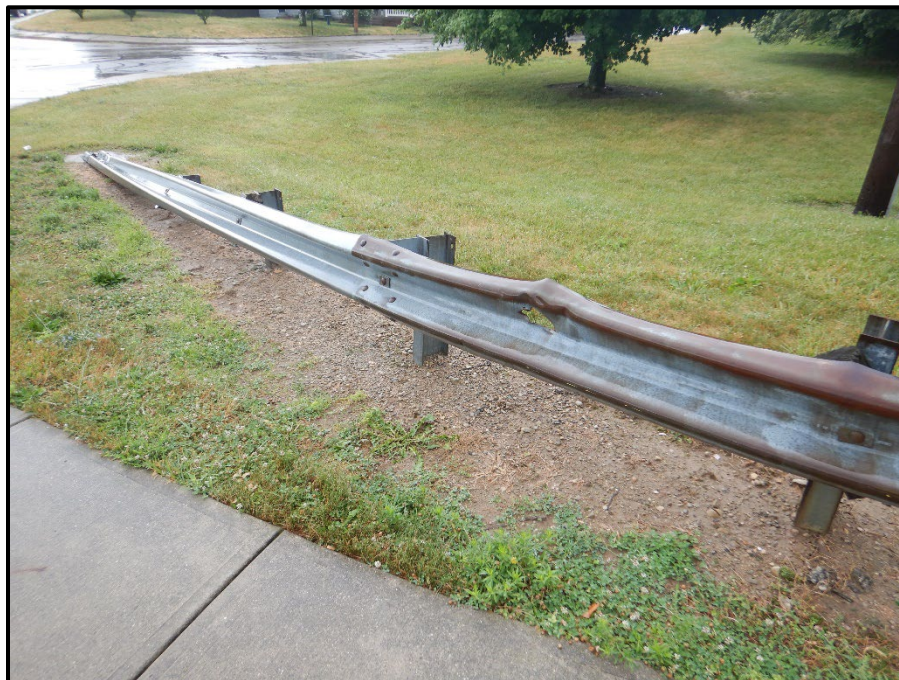
Photo 36 – Looking northwest at the northwest approach guardrail. Note: turn down end treatment.
