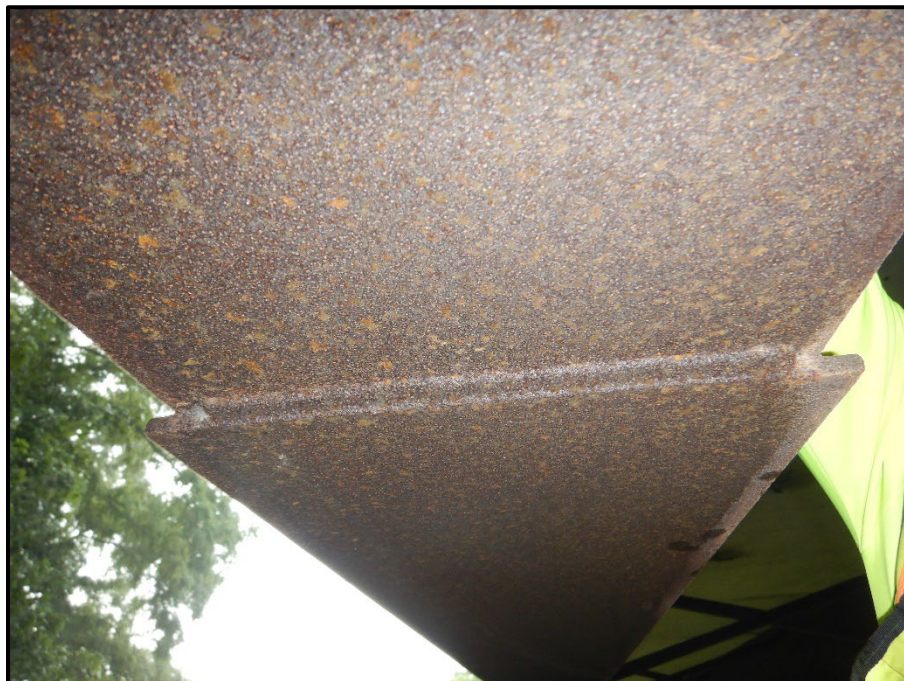
Photo 16 – Looking east at the moment plate on the bottom flange of beam A in span 1.
