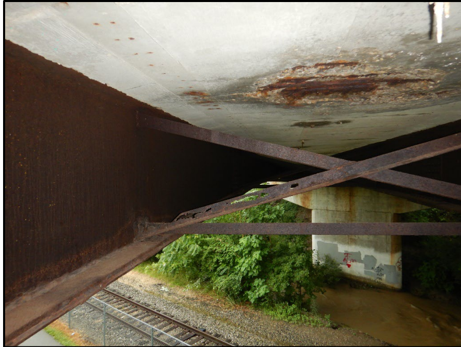
Photo 23 – Looking at span 3 intermediate cross-frame 10 between beams B and C near the Center Pier. Note: bottom of concrete deck spall and full depth corrosion holes exist in the cross-frame diagonal due to flow from the asphalt drain.
