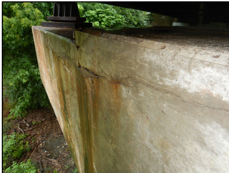
Photo 32 – Looking south at the south end, east face top corner of the Rear Pier between beams D and E. Note: 2-foot-wide x 4-foot-long x 16-inch-tall delamination caused by asphalt drain located directly above the cap.
