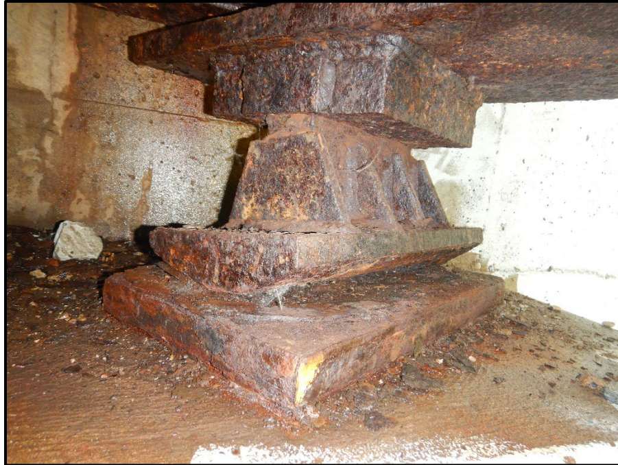
Photo 25 – Looking northwest at the beam A rocker bearing at the Rear Abutment. Note: laminar corrosion with up to 1/8 inch loss to the masonry plate and bearing interface.
