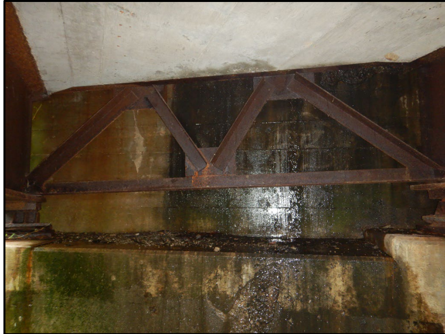
Photo 13 – Looking east at the end cross-frame between beams A and B at the Forward Abutment. Note: heavy surface corrosion exists on the end cross-frames due to water infiltration through the deck joint.
