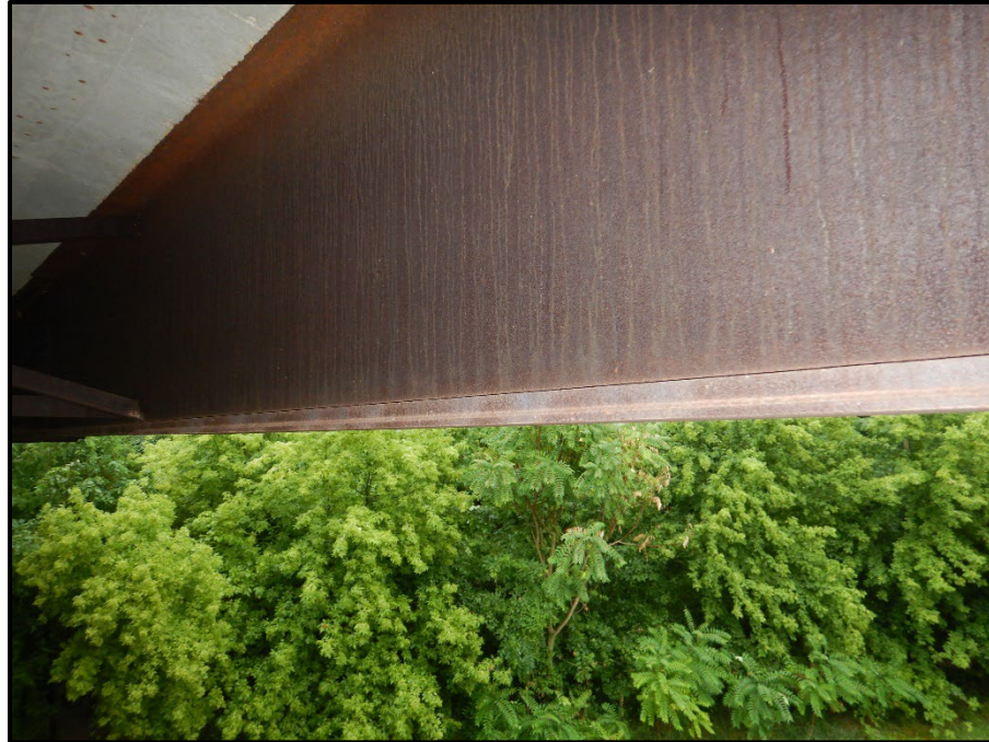
Photo 17 – Looking southeast at beam E in span 3. Note: moment plates are wider than the bottom flange.
