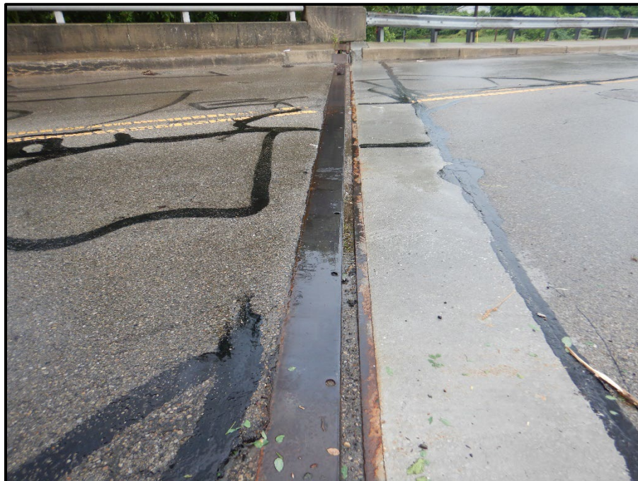
Photo 12 – Looking south at the sliding plate joint over the Forward Abutment. Note: soil and debris are accumulating in the joint.
