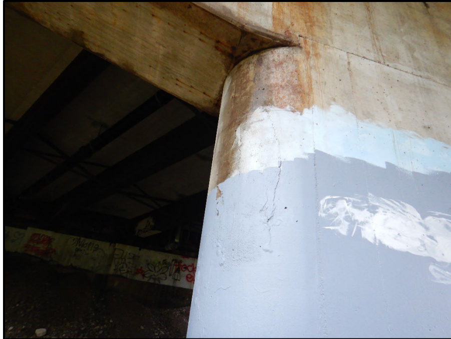
Photo 33 – Looking west at the south end of the Rear Pier wall. Note: 4-foot-tall x 2-foot-wide delamination caused by an asphalt drain discharging onto the top of the pier cap.
