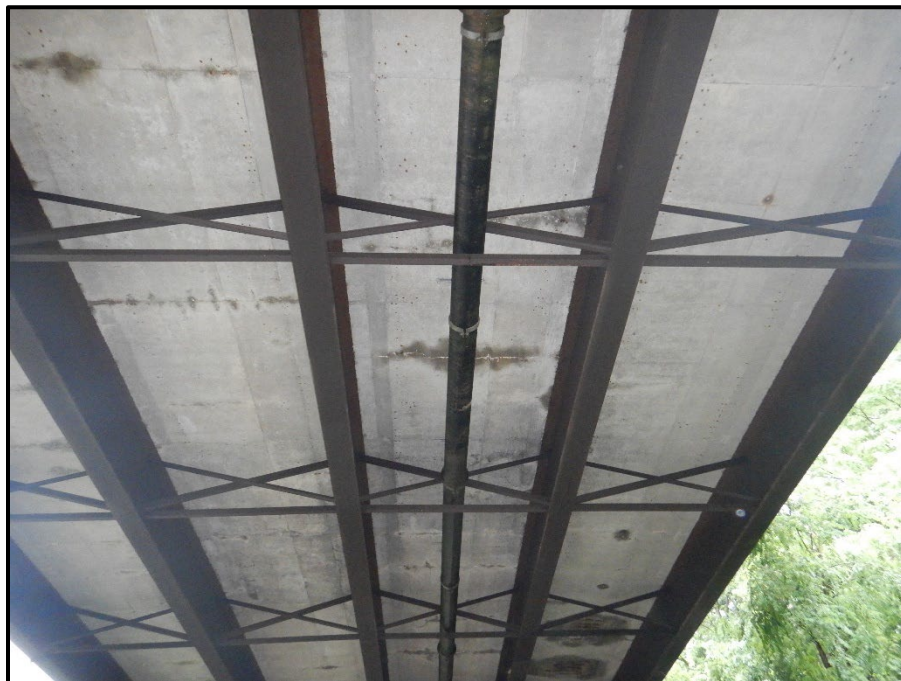
Photo 26 – Looking east at the water pipe running between beams C and D.
