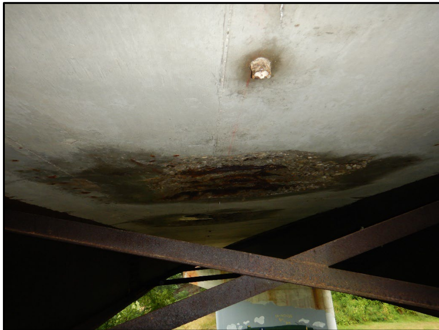
Photo 4 – Looking west at the underside of the deck in span 3 bay 4 near the Center Pier. Note: two 5-foot x 5-foot spalls with exposed reinforcing steel in the underside of the deck.
