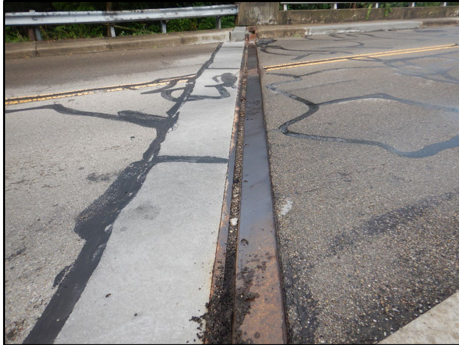
Photo 11 – Looking south at the sliding plate joint over the Rear Abutment. Note: soil and debris are accumulating in the joint.
