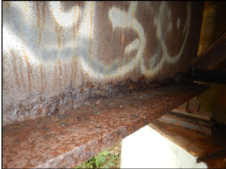
Photo 15 – Looking southwest at span 1 beam E at the Rear Abutment. Note: laminar corrosion typical on the end 4 feet the steel beams at both abutments.
