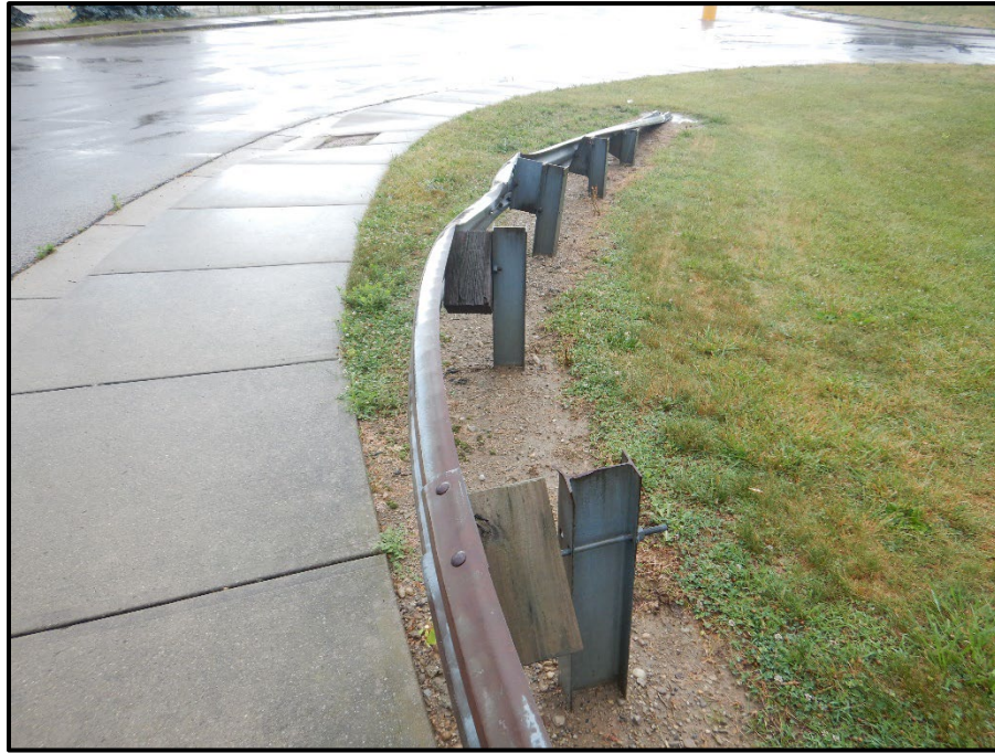
Photo 37 – Looking west at the northwest approach guardrail. Note: 5-foot-long section of impact damaged guardrail and multiple twisted and loose timber block outs.
