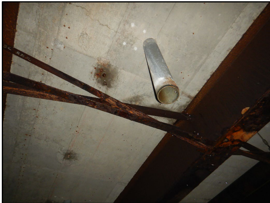
Photo 22 – Looking west at the scupper drain and asphalt drain in span 4 between beams D and E at cross-frame 17. Note: asphalt drain is directly over intermediate cross-frame and drainage flows onto diagonal member and down to the bottom flange of the beam.
