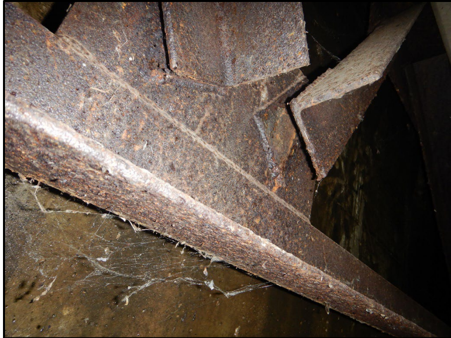
Photo 21 – Looking east at the end cross-frame between beams B and C at the Forward Abutment. Note: broken diagonal angle weld.
