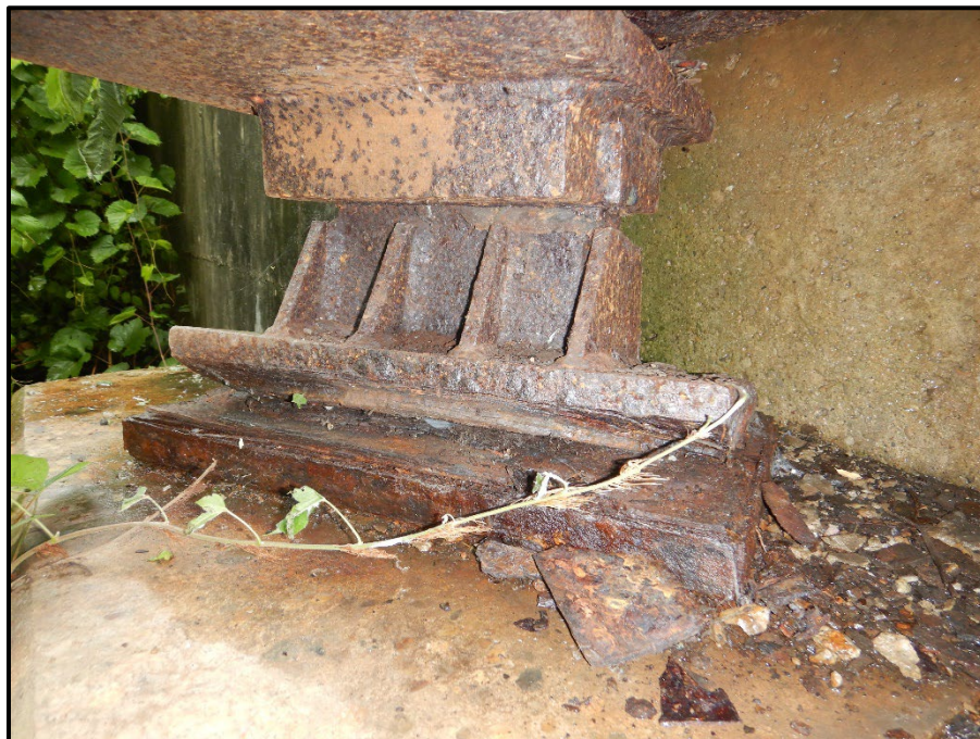
Photo 24 – Looking north at the rocker bearing under beam A at the Forward Abutment. Note: laminar corrosion exists to the masonry plate due to a leaking expansion joint.
