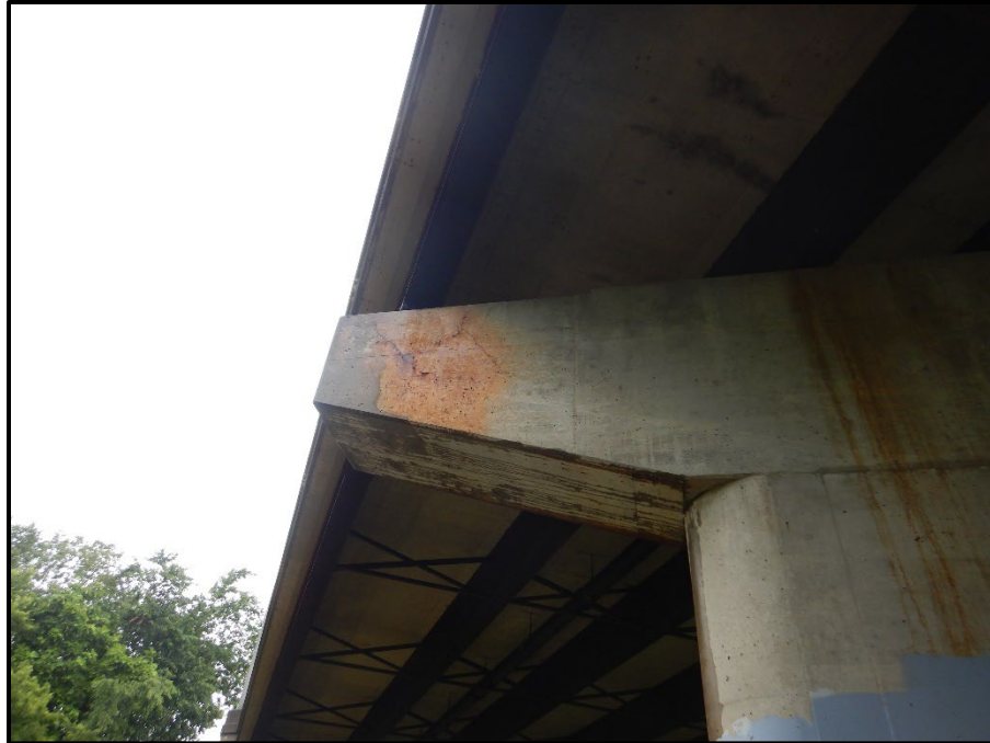
Photo 31 – Looking west at the south end, east face of the Center Pier cap. Note: multiple shear cracks emanating from the beam E bearing.
