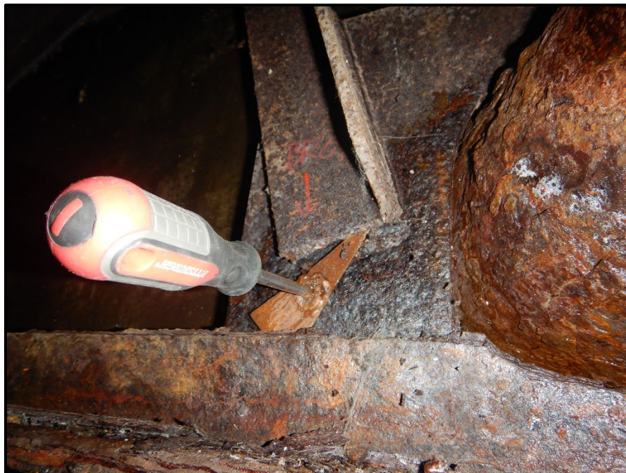
Photo 20 – Looking east at the end cross-frame between beams C and D at the Forward Abutment. Note: broken diagonal angle weld.
