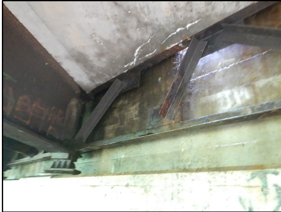
Photo 19 – Looking east at the end cross-frame between beams D and E at the Forward Abutment. Note: missing diagonal angle.
