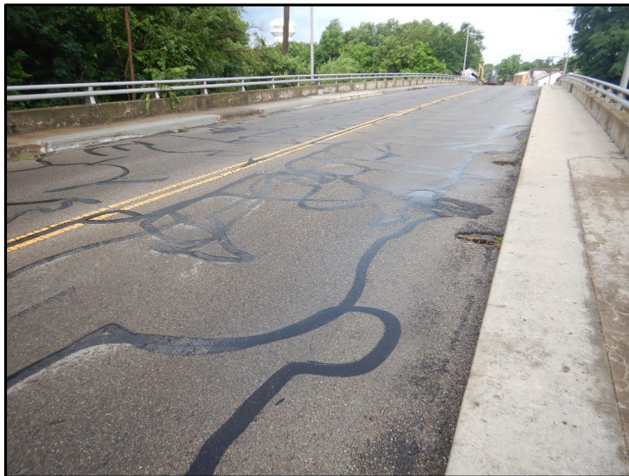
Photo 6 – Looking southwest at the typical wearing surface condition in span 1. Note: sealed map cracking throughout. Multiple locations of concrete sidewalk repair throughout all spans.
