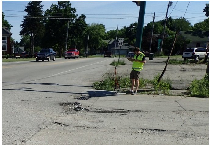
Photo 5: Deteriorated Gas Station Driveway
