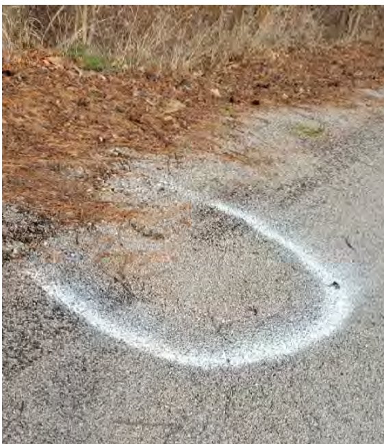
Photo 1: Typical Edge Deterioration
