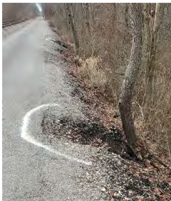
Photo 2: Major Edge Deterioration at STA. 849+20
