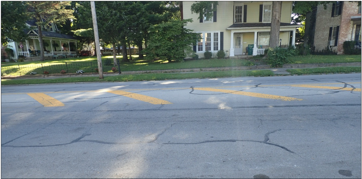
Photo 1: Faded Median Pavement Markings North of Washington Avenue & Gwynne Street
