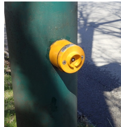
Photo 12: Push Button with No Cover at Oakland Street
