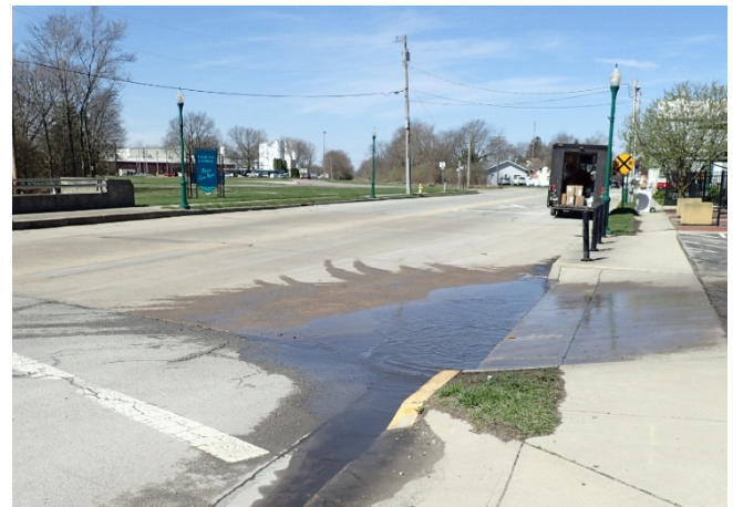
Photo 8: Standing Water at Coffee Depot House Driveway
