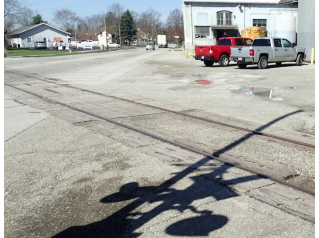
Photo 9: Wide Pavement at Premier Feeds
